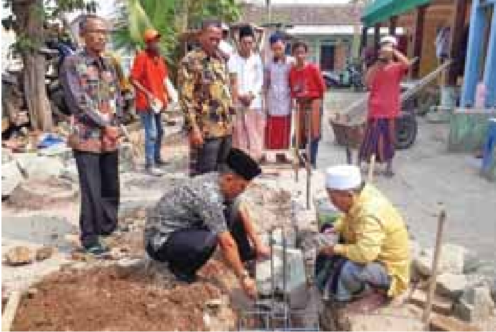
Groundbreaking ceremony of the SANITREN Program at Miftahul Huda Husmaniyah Pesantren at No. 13, Kayu Agung Village, by the Sepatan Subdistrict Head, Tangerang 2 .
